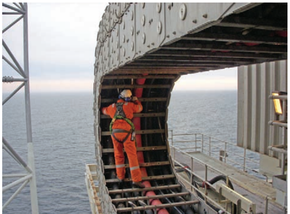
Inspection of hoses in Drag Chain performed by one of our service technicians.
